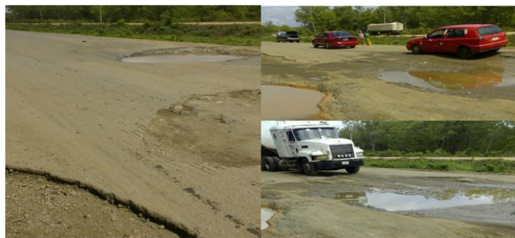
Figure 2.0 Failed portions of Ajaokuta-Itoke Road.
