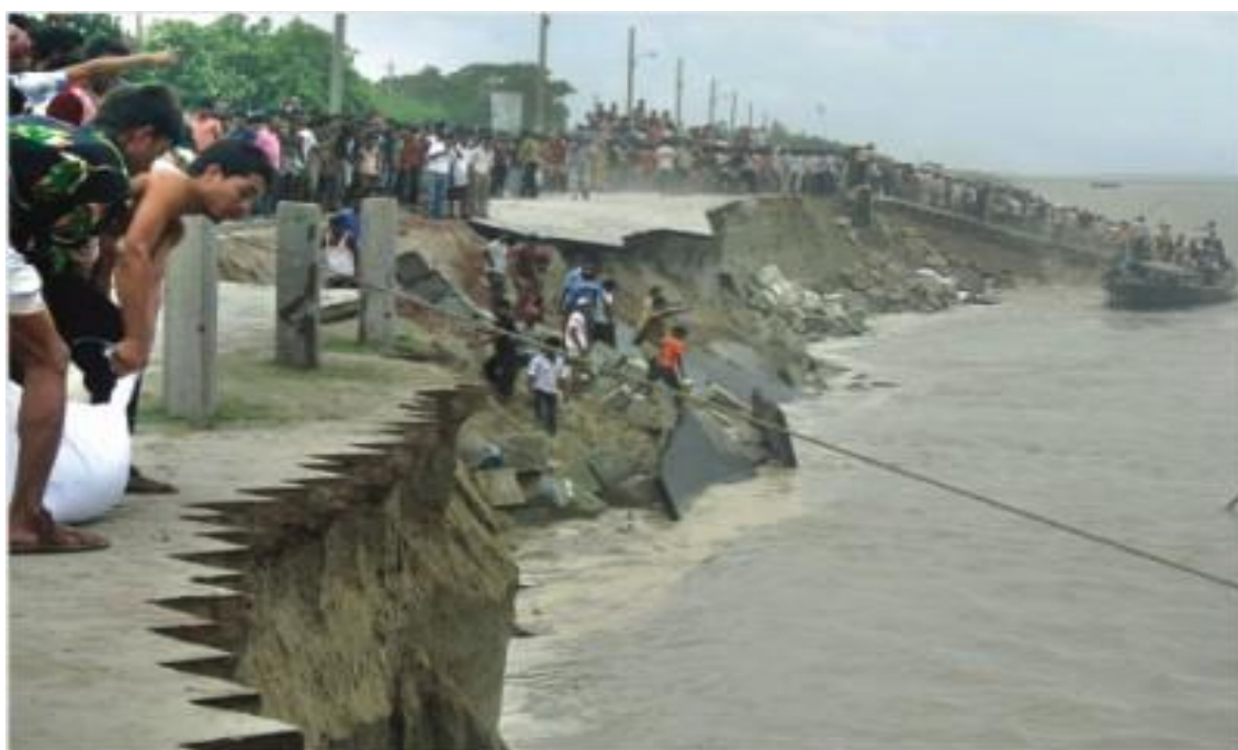
Fig. 2. River Embankment Broken Shirajganj Area (Jamuna River Side).
