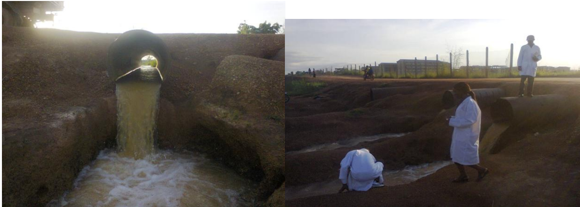
Plates 5&6. Underground storm channelization pipes at project site
