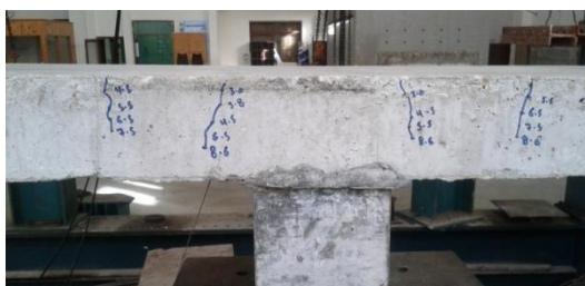
Fig. 3. Crack pattern of specimen S-20-85 after preloading and before strengthening.
