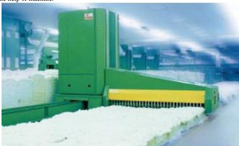
Fig. 3: Blow Room Department
